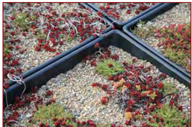
Other modular systems may have exposed lips, making them vulnerable to photodegradation and allowing for warm or cool air to escape from the building below.
