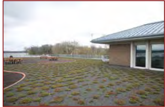
Day1: Conventional / Built in Place systems may look like this and be prone to weed infestation.
